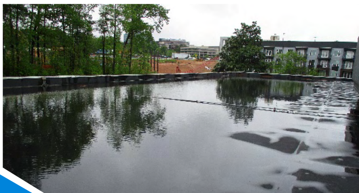
Figure 2. View of significant ponding on roof due to clogged roof drains with no overflow provisions. Photo by Christopher W. Giffin, F-IIBEC, RRC, AIA, NCARB
