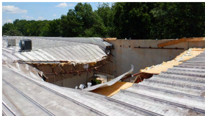
Figure 3. View of collapsed warehouse building roof due to excessive ponding water. Photo by Christopher W. Giffin, F-IIBEC, RRC, AIA, NCARB
