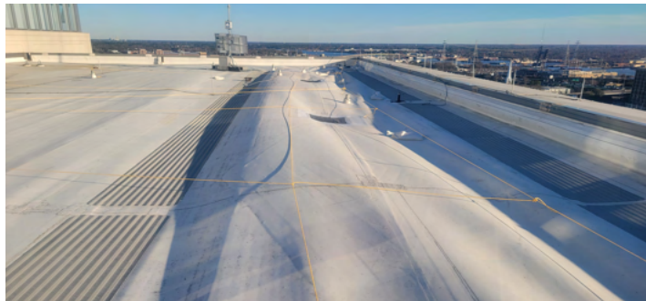
Figure 4. View of roof damage resulting from insufficient wind uplift resistance. Photo by REI Engineers Inc.
