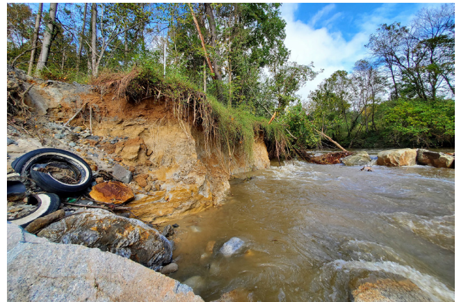
Collapsed bank of Salem Creek (before restoration)
